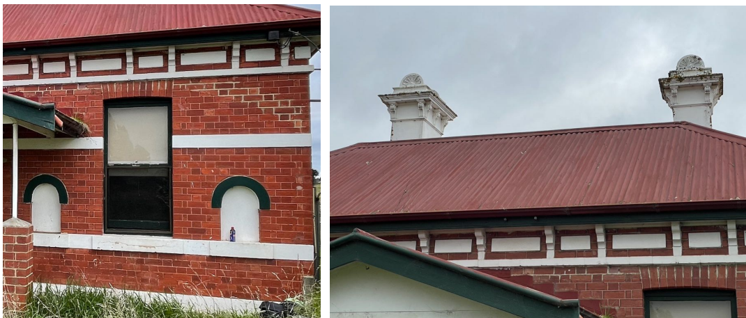
Figure 4: Detail showing eaves and rendered band decoration, segmental arch window and niches, and evidence of original verandah profile, and chimneys at right (Source: David Helms, 2023).
