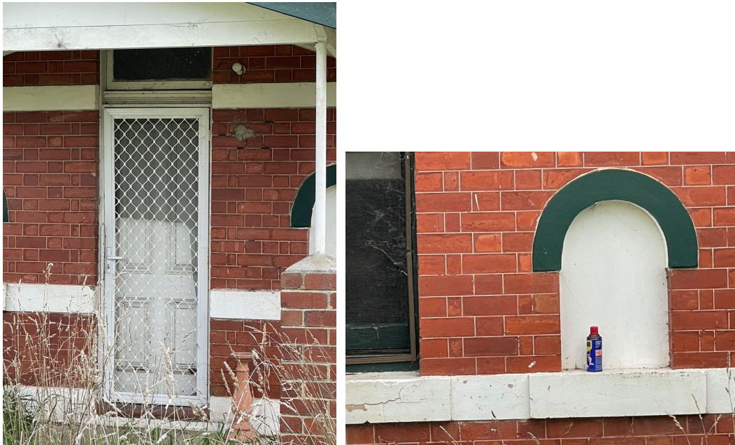
Figure 5: Detail of front door, niche and cills, and wall showing white tuckpointing (Source: David Helms 2023)
