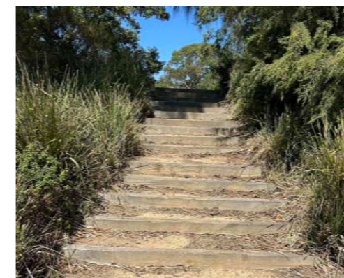
C The stairs and viewing platform are in poor condition and need improvement
