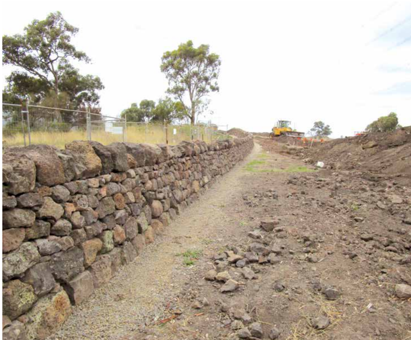
Reconstructed Dry stone wall along Findon Road, South Morang. Source: Colleen Lazenby
